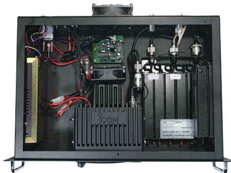
CY-F121S Series Repeater, inside top.
